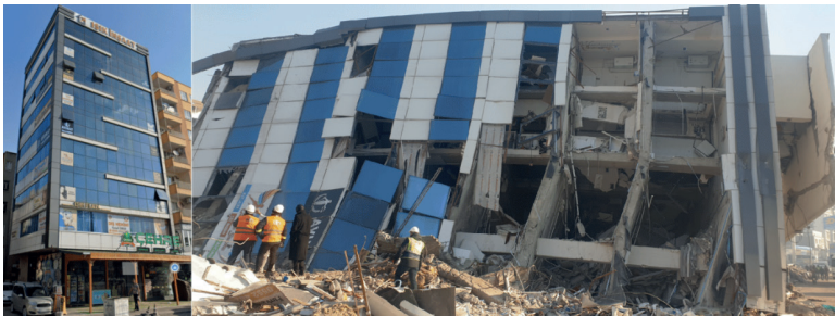
Figure 7. Collapse of a building as a result of the 2023 Kahramanmaraş earthquakes (Mertol et al., 2023)
