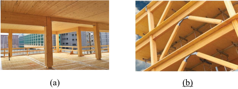
Figure 4. (a) Wooden frame system with glulam column-beams and NLT flooring (Shahnewaz et al., 2023), (b) cross braced wooden frame system (Iqbal, 2021)
